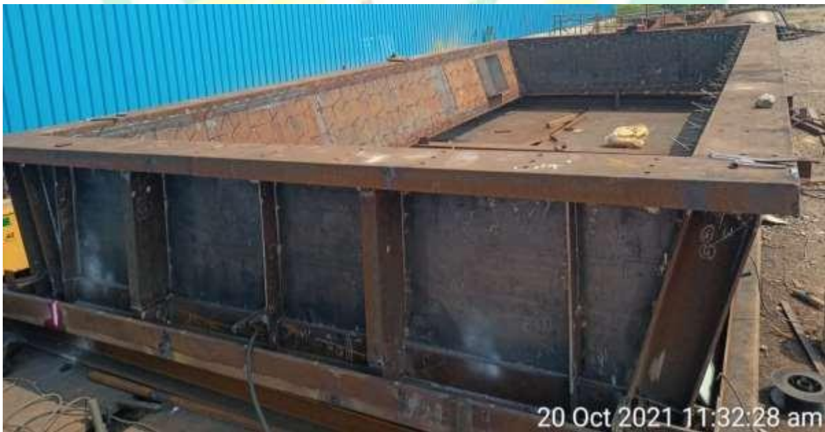
01-H-201-PRIMARY REFORMER SHOP DRAWING HOT FLUE GAS DUCT FGD-01, FGD-02 & FGD-03, GPUFP – BANGLADESH
